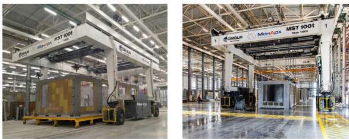
Fig. 3. Technological portal conveyor ( Q=100 t) for conveyor assembly of MonArch Group modules
