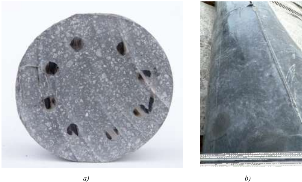
Fig. 3. Concrete compaction quality: a — reinforced concrete core in section; b — lateral surface of the reinforced concrete core
