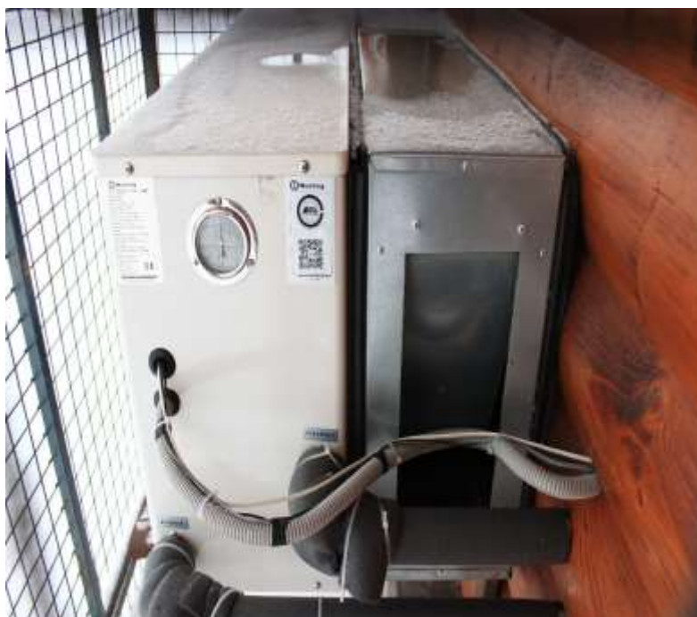
Fig. 6. Air mixing chamber [15] and an ASHP installed in a low-rise residential building in the Ivanovo region
